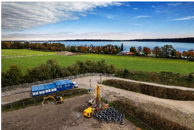
(1) Bauer Resources is constructing a geothermal probe system for a high school in Diessen with a spectacular view of Ammersee Lake.
