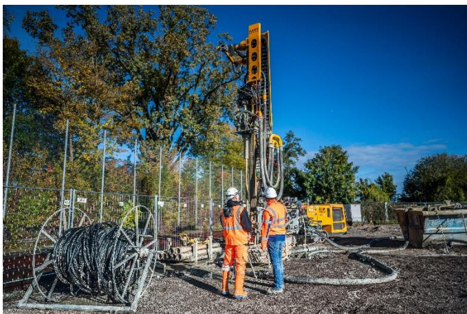
(2) Using two powerful KLEMM KR 805 rigs, two drilling teams executed roughly 5,700 drilled meters.
