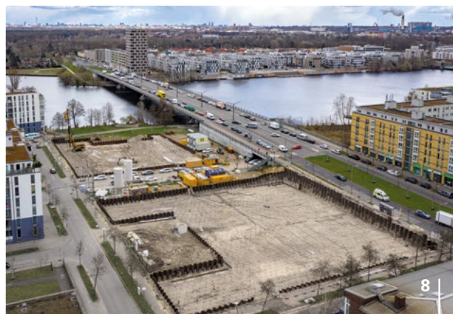
7 | Munich Along with other joint JV partners, Bauer is involved in the construction of the 2nd Stammstrecke (Home Line) in Munich, a massive infrastructure project. The initial excavation pit for the tunnel boring machine at the Donnersberger bridge has already been completed.
