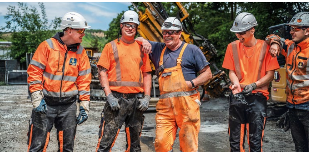
Harnessing their full team power and precision, the experts from Bauer Spezialtiefbau master all the challenges.
