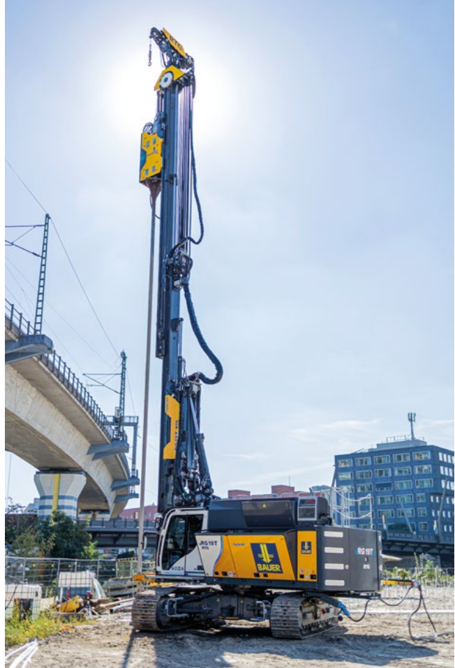
Successful first operation of the eRG 19 T hybrid on a project at Friedrich-Krause-Ufer in Berlin.
