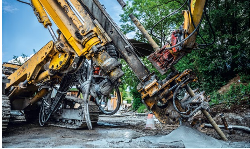
To safeguard the lock, Bauer executes the necessary grouting work with the configured KLEMM KR 806-2DB.
