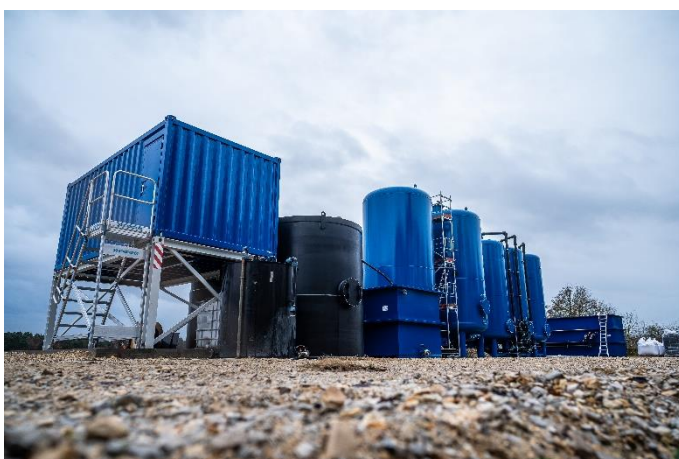
(1) Bauer Resources constructed a customized groundwater treatment plant on a military site in Manching.
