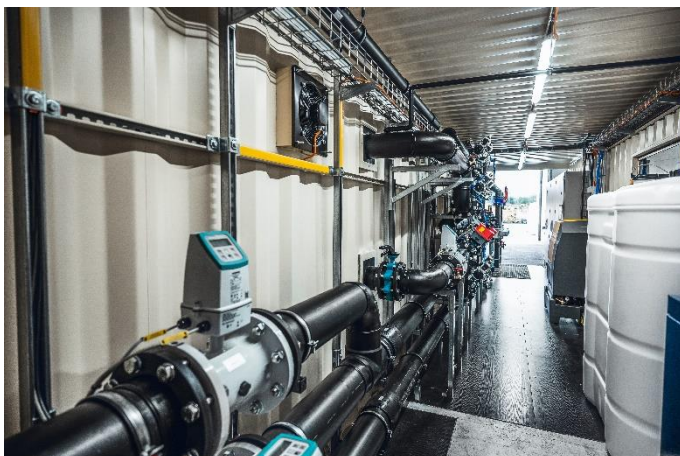
(3) The plant treats around 150 m 3 of groundwater polluted with PFAS per hour.
