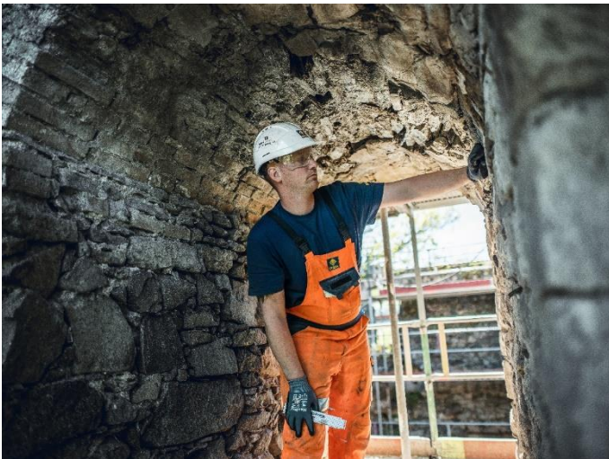
(3) During the rehabilitation work, approximately 2,400 m 2 of joints in the basalt wall structures were restored.
