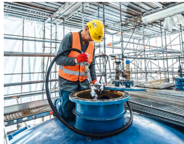
Bauer Resources produces groundwater treatment plants from small to large.
