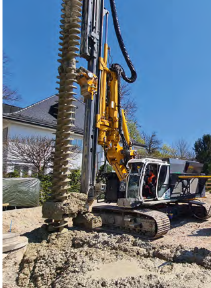
A Bauer Spezialtiefbau project in Munich, in which Bauer Resources was also involved, received the DGNB Certificate for Sustainable Construction Sites.
