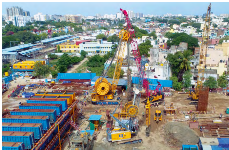
In the Indian metropolis of Chennai, Bauer is involved in subway expansion work. More than 15,000 m 2 of diaphragm wall were installed for the Chetpet Metro Station.
