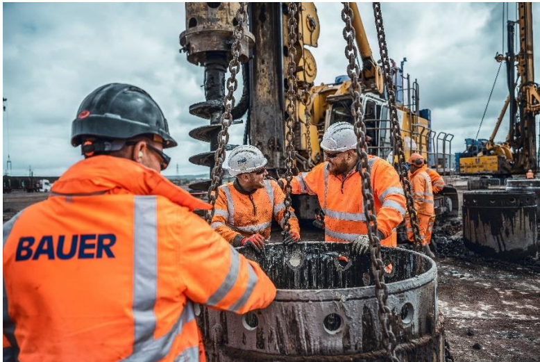
(1) A strong team at work: Roughly 1,500 bored piles and 5,500 CFA piles form the foundation for the planned monopile manufacturing facility.
