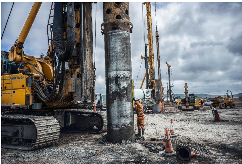
(2) Thanks to precision and good planning, the specialist foundation engineering work was successfully concluded in just 14 months.
