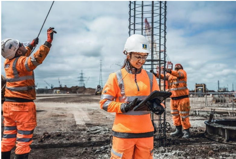
(3) Site Engineer Vidhya Brahmalingu ensures good planning and organization on the construction site.
