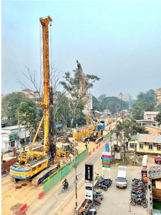
(1) Bauer India is installing a total of 150 piles for the construction of a four-lane flyover.
