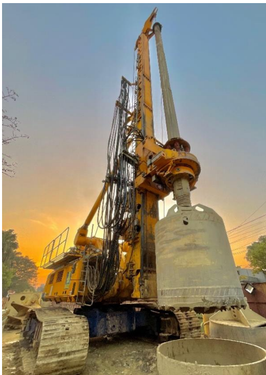
(2) The installation of piles with a diameter of 2,000 mm in extremely cramped conditions was anything but routine.
