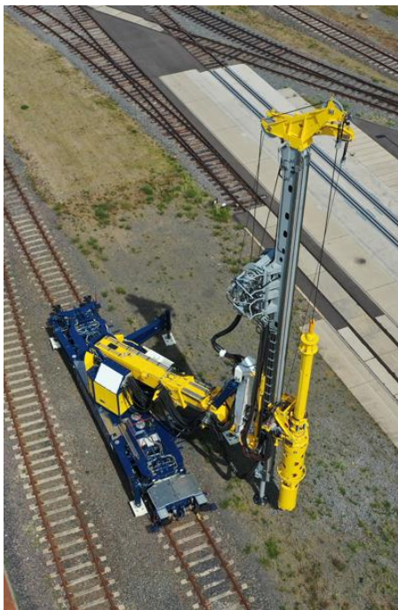
(1) The overall system consists of the base carrier with leader based on a RTG RG 18 S.
