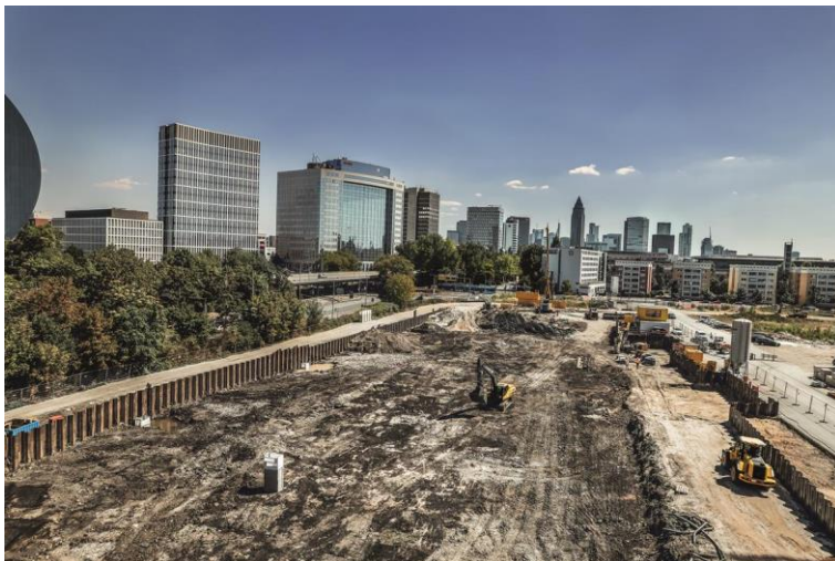
(1) Since April, the Bauer Umwelt Division of BAUER Resources GmbH has been constructing a 15,000 m 2 excavation pit on a former military site in Frankfurt am Main.
