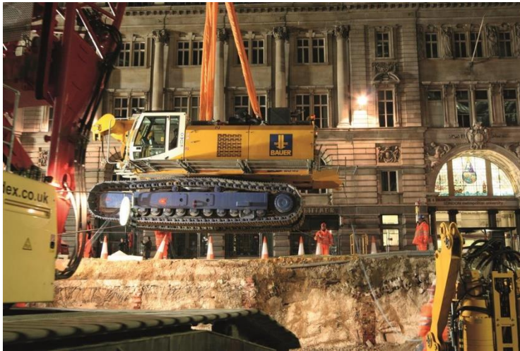
(2) The core of the specialist foundation engineering work for the Moorgate Shaft at Liverpool Street station was the construction of a 60 m deep shaft.
