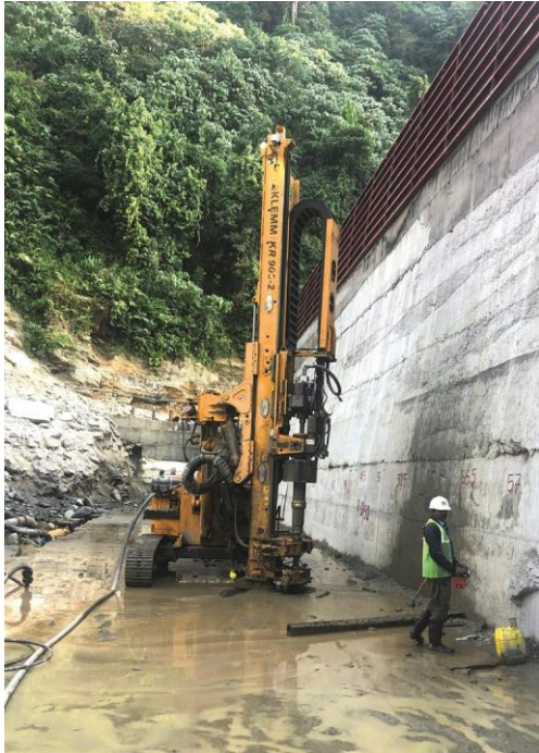
A KLEMM KR 909 is being used for the drilling and injection work. © BAUER Group
