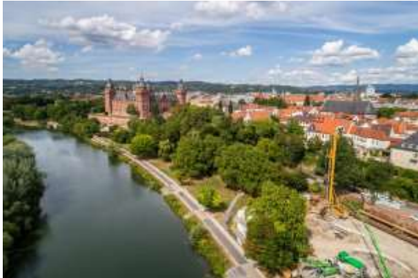
(1) A BAUER BG 40 constructs CFA piles in the German city of Aschaffenburg – in the background: the picturesque Johannisburg castle.
