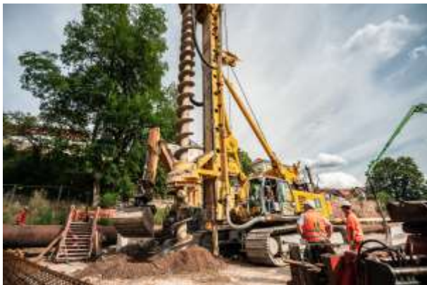
(2) BAUER Spezialtiefbau GmbH constructs the retaining structure using a secant pile wall up to a depth of 24 m.
